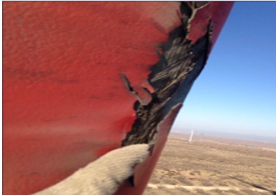
Fig.3 Blade Lightning Strike Damage
